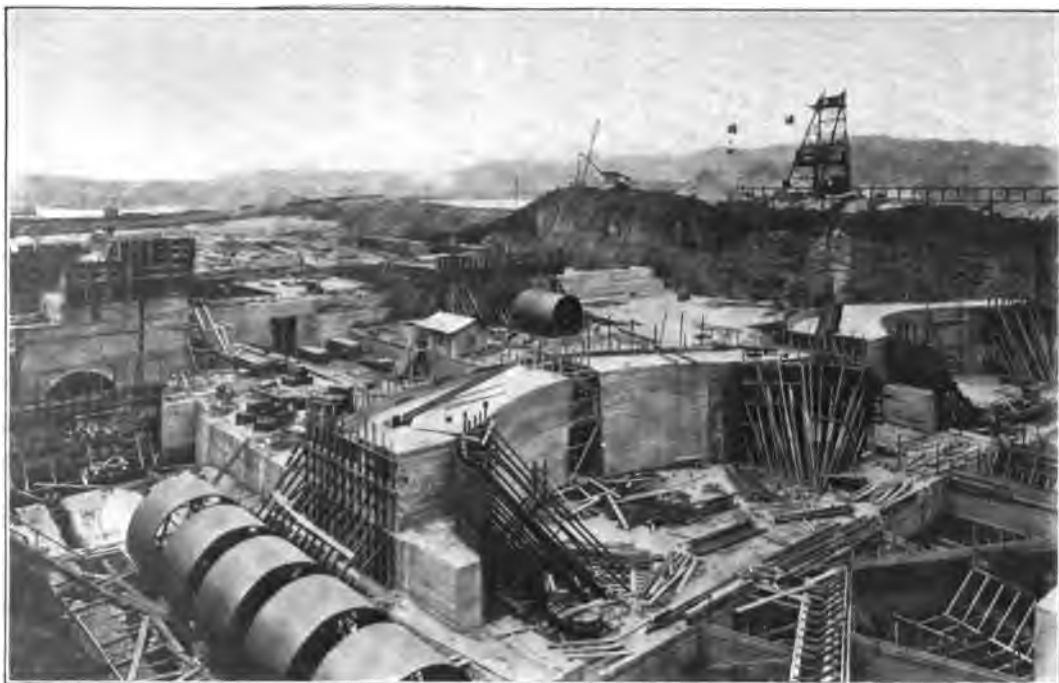
FOREBAY AND LIFT SILL, LOOKING SOUTH, FROM EAST WALL, GATUN LOCKS, MARCH 15, 1910.
